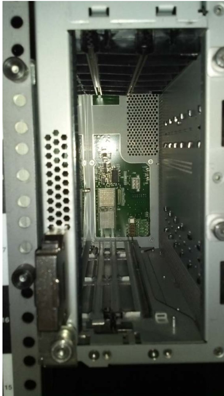
Figure 12-36. EEB removed - vacant slots
