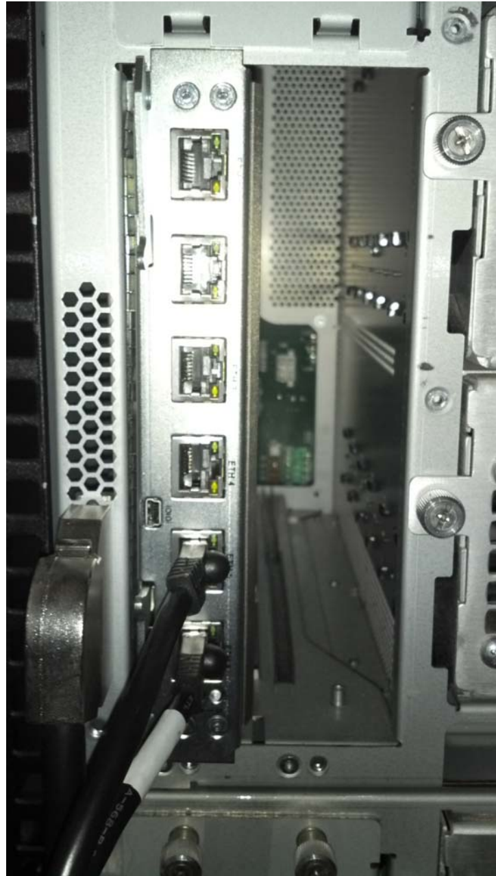
Figure 12-34. EEB with small cover plate to the right removed
