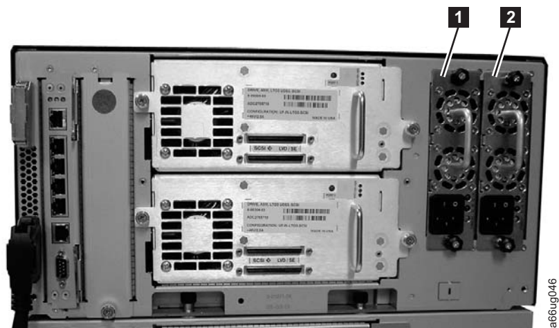
Figure 12-31. Power supplies in a control module
