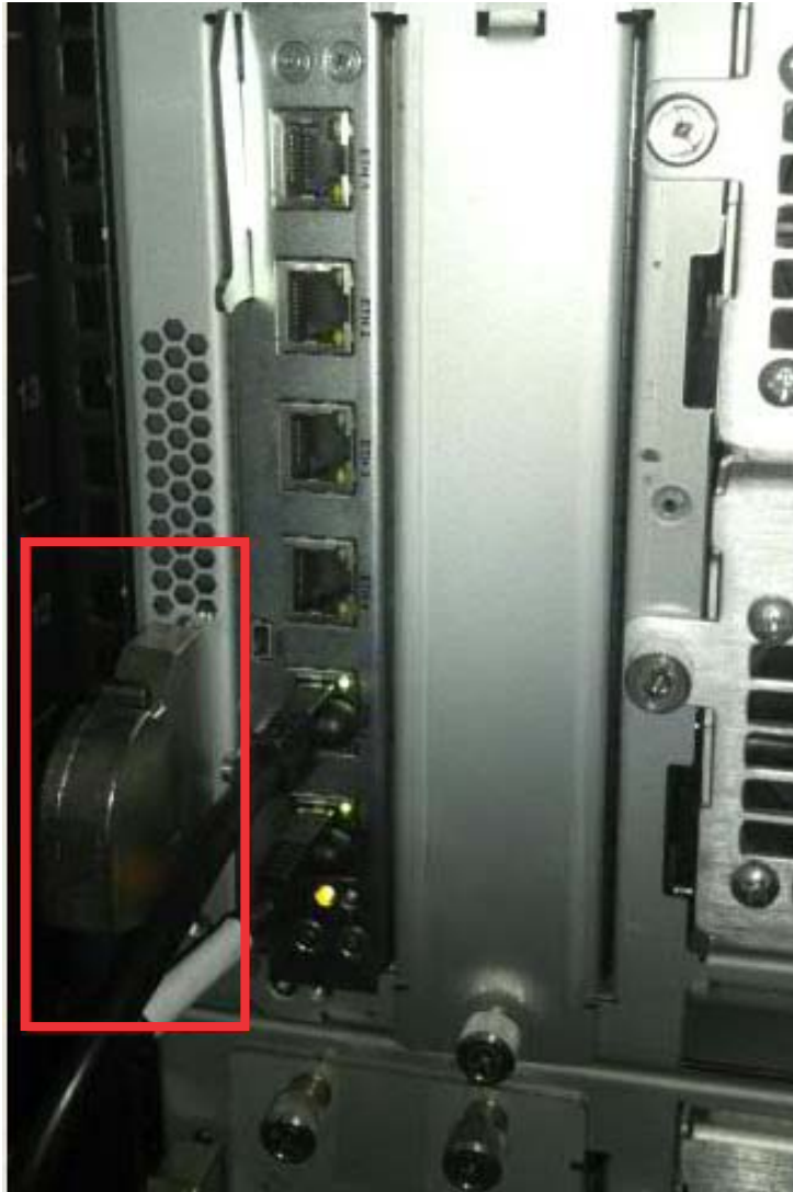
Figure 12-43. Replaced Module Communication Terminator
